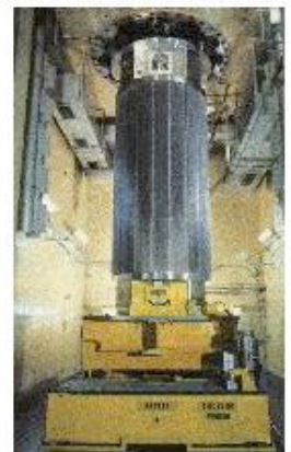
Figure 2: Dry fuel unloading
